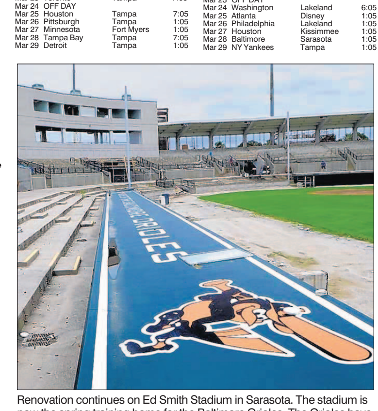
Renovation continues on Ed Smith Stadium in Sarasota. The stadium is now the spring training home for the Baltimore Orioles.
